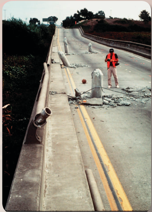
Figure 12. Bridge damaged by earthquake – note pillars popping through the road surface (image by U.S. Geological Survey).
