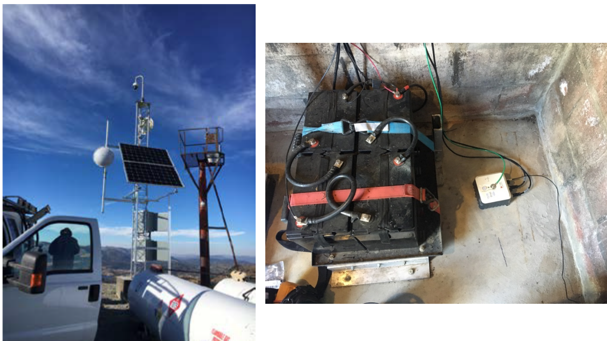
Figure 2. (left) Mt. Lincoln (Sugar Bowl Ski Resort) communication hub/fire camera with back-propane generator that supports microwave communications in the Truckee EEW region. This site was funded through ALERTWildfire efforts to monitor extreme weather events in the Sierra Nevada. (right) Big Hill EEW ETNA2 indoor installation at ALERTWildfire camera site. This AC grid-powered site incorporates a 24V battery backup system to power the equipment through PSPS events and unplanned lapses in power.
