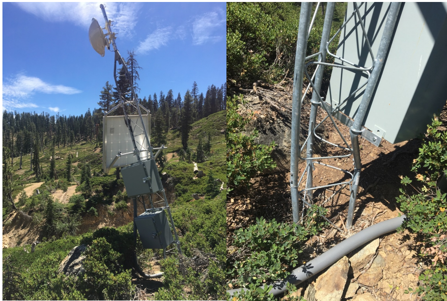
Figure 3. Sierra Butte (SBT) Rohn-25 tower failure to 2018-2019 winter storms.
