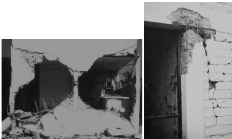
Figure 17. Damage to confined masonry buildings in the 1985 Llolleo, Chile earthquake 1
