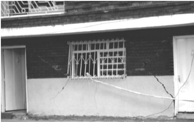
Figure 21. Observed damage at the ground floor of a confined masonry building in the 1999 El Quindio, Colombia earthquake (note that the tie-columns around the openings are missing) 8
