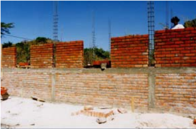
Figure 2. Confined masonry construction in Slovenia, with the walls built using hollow clay tiles (top) 2 and El Salvador (bottom) 3 (note the walls built using burnt clay bricks)
