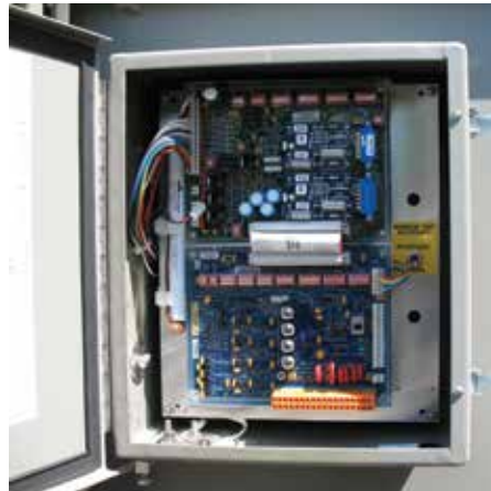
Figure 16. TPG control with SCADA shown.
