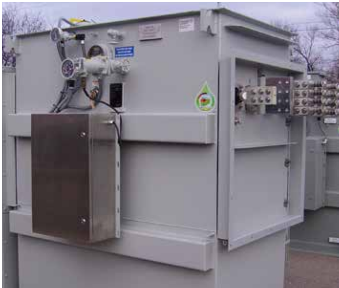
Figure 13. Substation transformer with customer-specific coordination and accessories.
