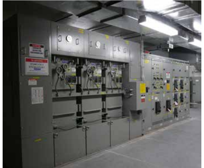
Figure 14. Triplex Indoor Power Center comprised of energy efficient and low noise single-phase substation transformers in a ganged setup.
