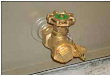
Figure 3. Drain valve with sampler.
