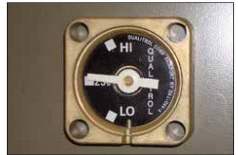
Figure 5. Liquid level gauge.
