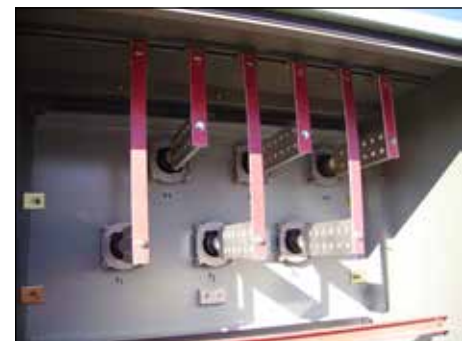
Figure 11. 12-pulse application with bushing supports.
