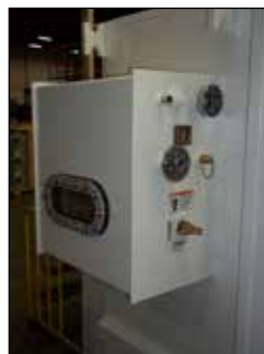
Figure 7. External visible break with gauges.
