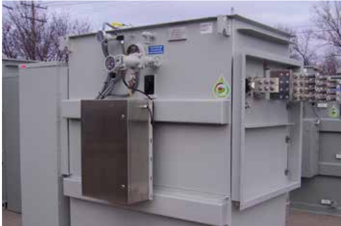
Figure 21. Substation transformer with customer-specific coordination and accessories.
