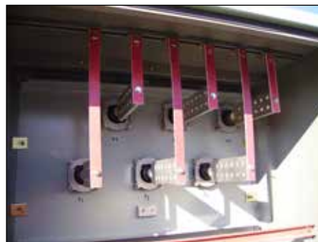
Figure 11. 12-pulse application with bushing supports.
