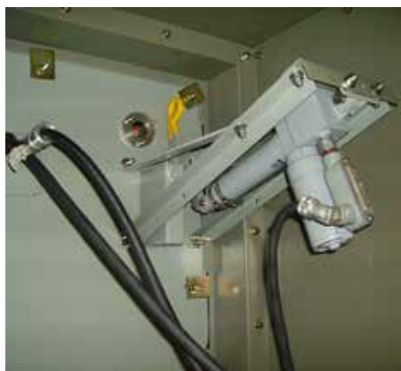
Figure 14. Motor-operator for open/close of vacuum fault interrupter (VFI).
