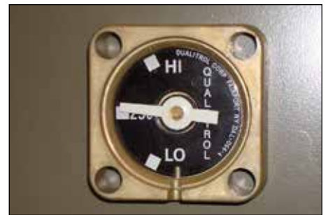
Figure 5. Liquid level gauge.
