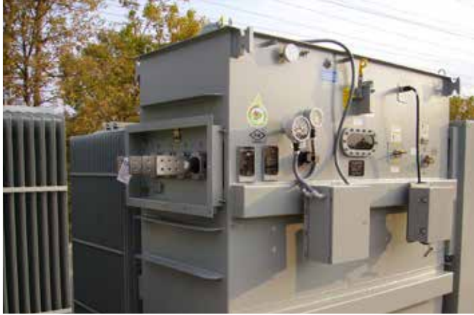
Figure 20. Substation transformer with visible break technology.
