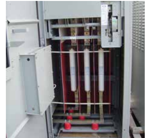
Figure 19. LIS—interior view showing power fuses.
