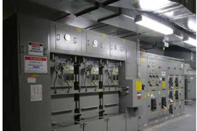
Figure 22. Triplex Indoor Power Center comprised of energy efficient and low noise single-phase substation transformers in a ganged setup.
