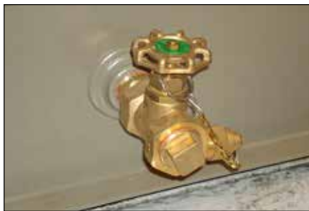
Figure 3. Drain valve with sampler.
