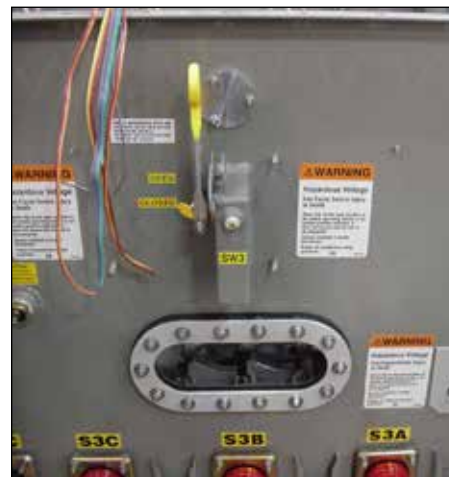
Figure 8. VFI transformer with visible break.
