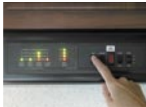
Central monitor panel.
