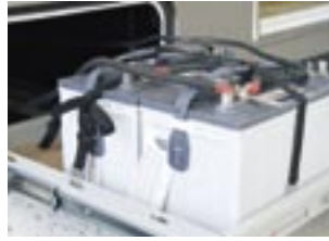
Auxiliary battery tray.
