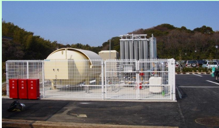
Installation for GHP in a Factory
