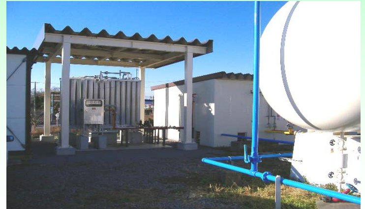
Installation for Community Gas Supply
