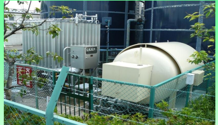
Installation for Boilers in a Factory
