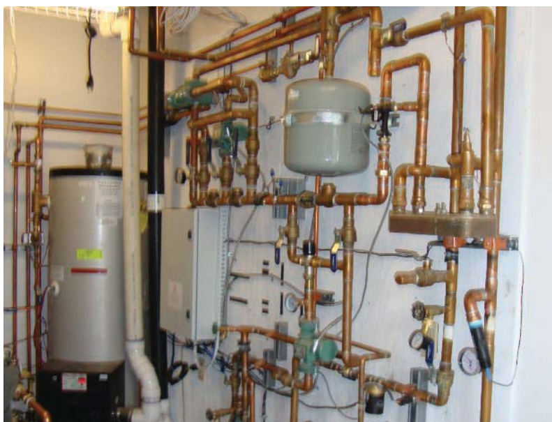
The piping design is a dual primary loop, where every source and every load is connected to one of the primary loops with two closely spaced tees. This piping arrangement allows heat to be delivered directly from any source to any load at any time, bypassing storage tanks when appropriate.
