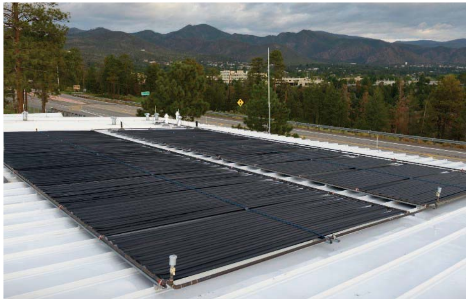
Sun Ray unglazed flat panels on the roof provide night sky radiant cooling (NSRC) to pre-cool the concrete floors in summer. On average, this provides the equivalent cooling of a 1-ton air conditioner running for four hours for just a few kWh of electricity.
