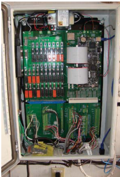
The SolarLogic Integrated Controller (SLIC) allows complete control, monitoring, and adjustment over all hydronic heating and cooling in the building, locally and remotely.
