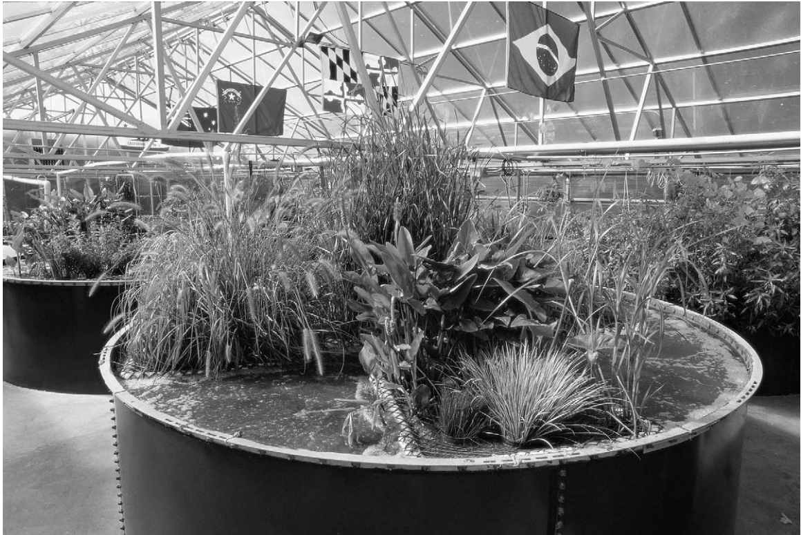
Fig. 2. Photograph of tank at the south Burlington, VT AEES. This planted aerobic tank is one of the first in a series of similar tanks used for treatment of municipal waste in Vermont. The roots of plants installed in racks on the top of the tank provide the necessary diverse microhabitats for effective and efficient treatment.
