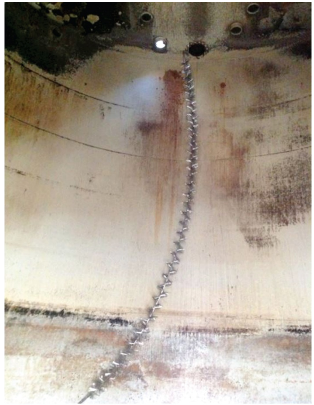
Figure 7. Example of in-tank static dissipater (source: Lightning Master Corporation). EERC BS56751.AI
