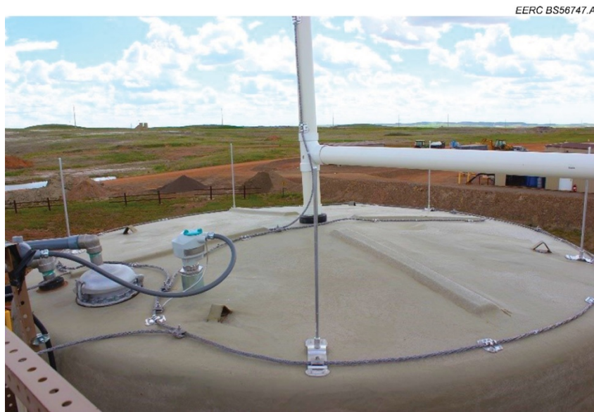
Figure 3. Example of traditional air terminals.
