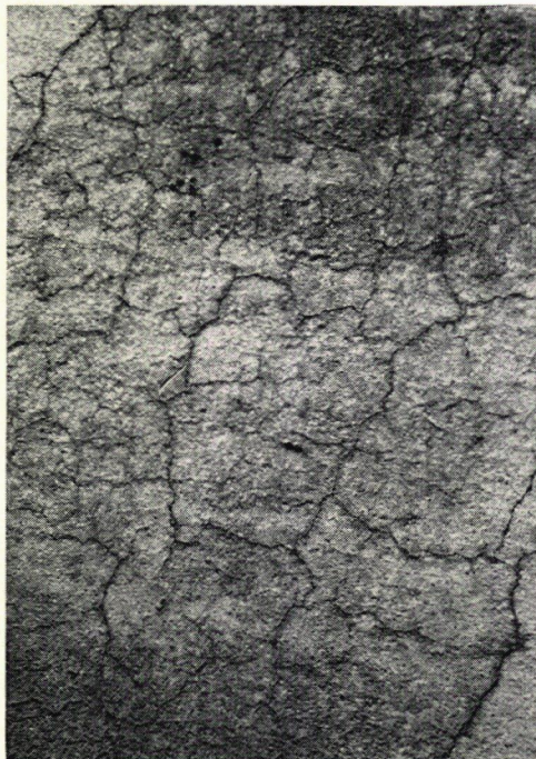
Figure 1. Typical map cracking in concrete made from sand gravel aggregate.
