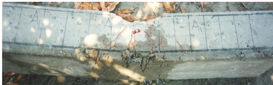
Figure 2 b: Shear Cracks on beam (A 1 ); Flexure Failure
