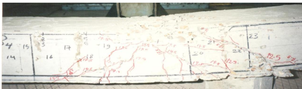
Figure 3 e: Shear Cracks on beam (B 4 ); combined flexure and shear failure
