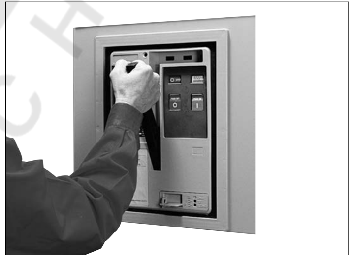
Figure 30. Circuit breaker closing springs being manually charged
