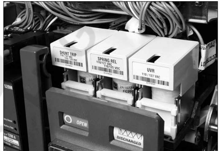
Figure 46. Shunt trip, spring release, and undervoltage release installed
