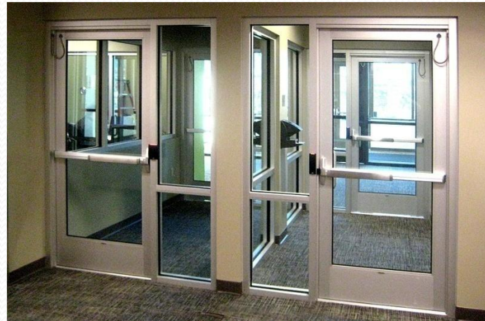
Mantrap Shield installed into two purpose-built airlocks
