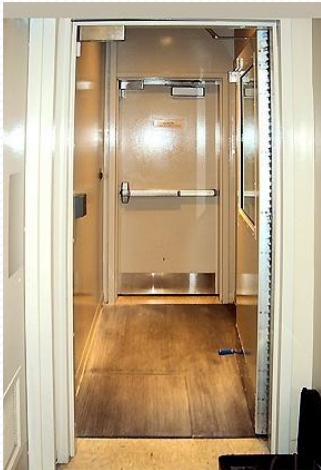
Mantrap Shield in airlock converted from a corridor
