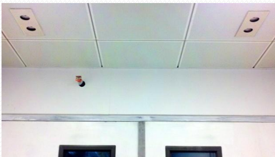
Typical Model DS200 installation in a drop ceiling.
