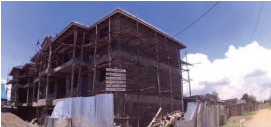
Ongoing construction of a residential apartment is contrary to the prescribed zoning. Source: © UN-Habitat
