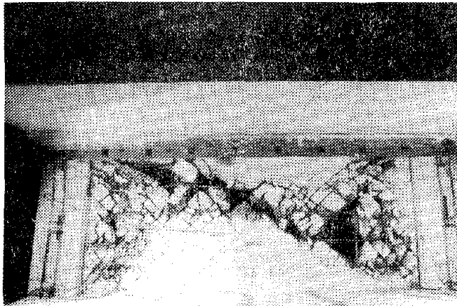
FIG. 4.58 FAILURE ZONE: THIRD-STORY WALL PANEL OF SPECIMEN SW7 R 2 . EXPOSED AND BUCKLED PANEL REINFORCEMENT. END OF TEST.
