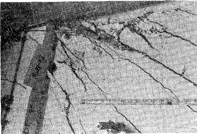
FIG. 4.56 SPALLING OF CRUSHED CONCRETE IN UPPER NORTH CORNER OF THIRD-STORY WALL PANEL OF SPECIMEN SW7 R 2 . LP 450.
