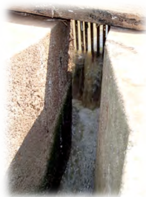
Figure 4: Screening at the municipally WWTP.
