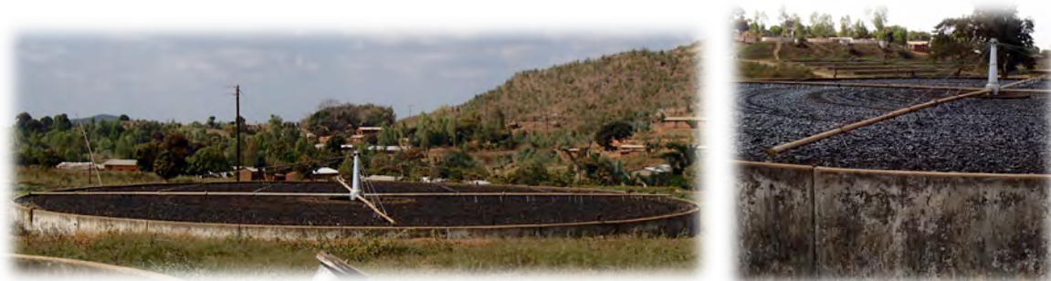
Figure 6: Biofiltration at the municipal WWTP.
