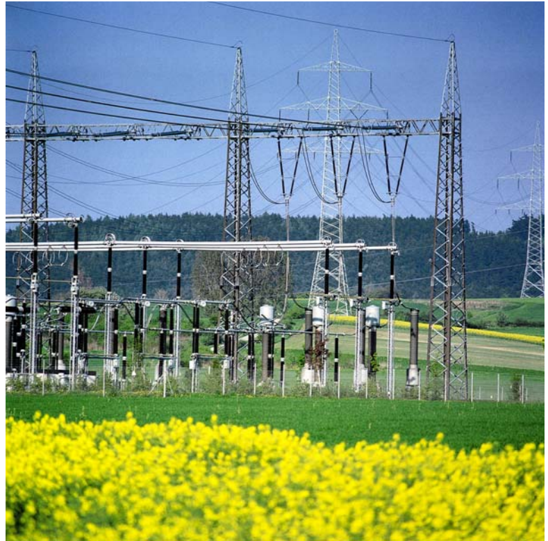
Fig. 1 400 kV outdoor switchgear
