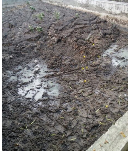
Poor filtration of sludge before intervention
