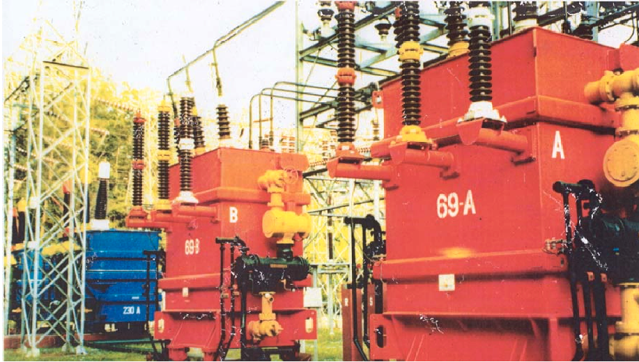
Figure 1.15: Substation power transformers.
