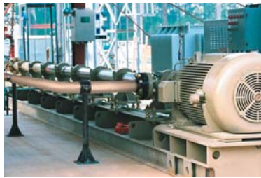
SP1000 CO 2 pipeline injection Mississippi, USA
