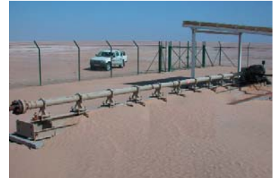
SP1000 waterflood injection installation Oman, Middle East
