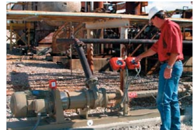
SP75 amine gas service application Texas, USA
