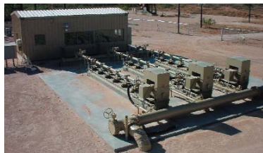
SP1000 (3) parallel water injection Texas, USA
