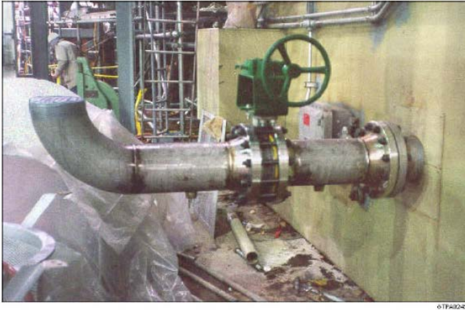
Figure 91. Inlet Air Heating Piping Running Through Enclosure Left Side Wall
