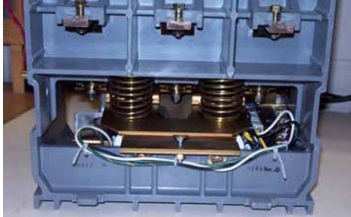
Figure 10 – Contactor (rear view) showing wires to be wire-tied
