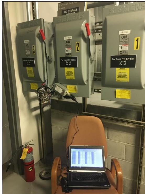
Photograph 1. Energy monitoring software connected to three-phase elevator circuit
