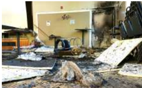
Fire damage in the ballroom. Photo credit Restore Oregon.
