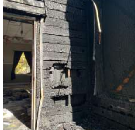
Where fire started at building’s rear corner. Photo credit Restore Oregon
