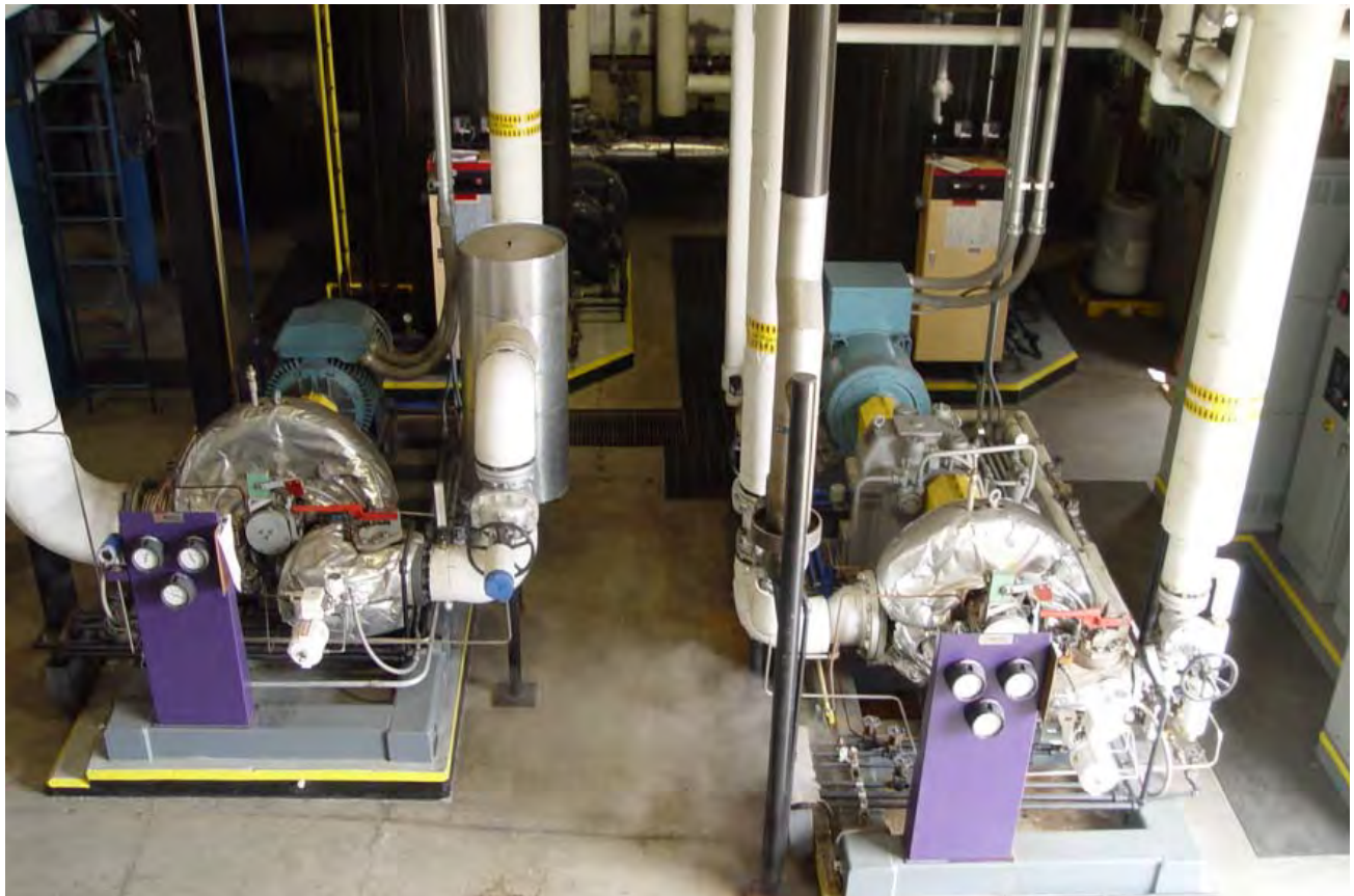
This biomass project included two STGs. The left STG is induction with a power of .257 MWe. The right STG is synchronous with a power of .260 MWe.
