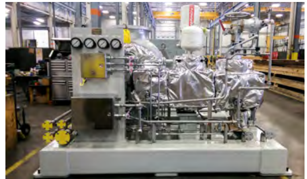
This 2.6 MWe synchronous generator was used for a CHP project.
