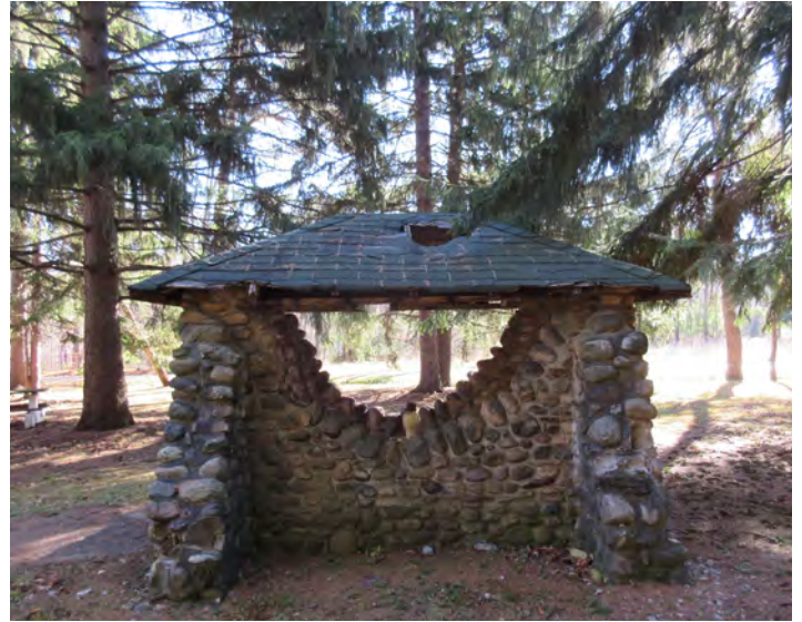
Pump shelter with hole in the roof
