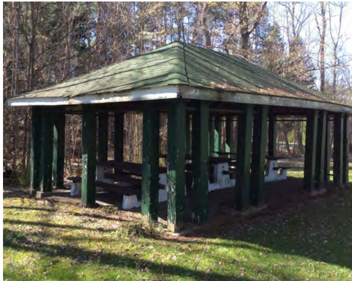
Shelter #117: Recommend demolition
