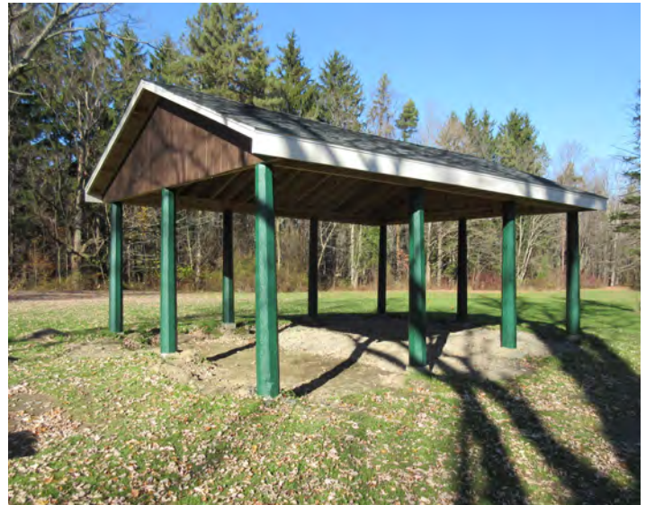
Shelter #13: Recommend demolition
