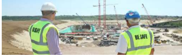
Collaborative planning resulting in a 4 week saving equating to £400K on the LD's.
