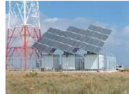
Solar powered cell tower
