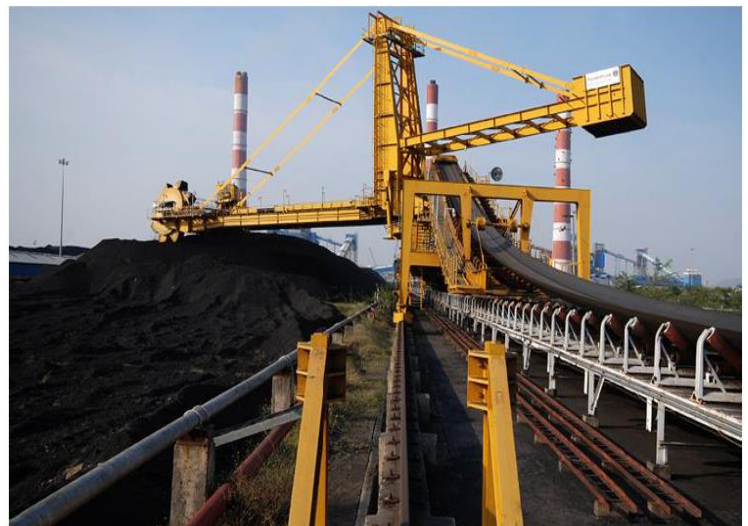
Figure 8:- Picture of Coal handling plant of NTPC Dadri
