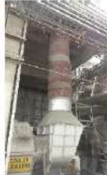
Entry at fan inlet
