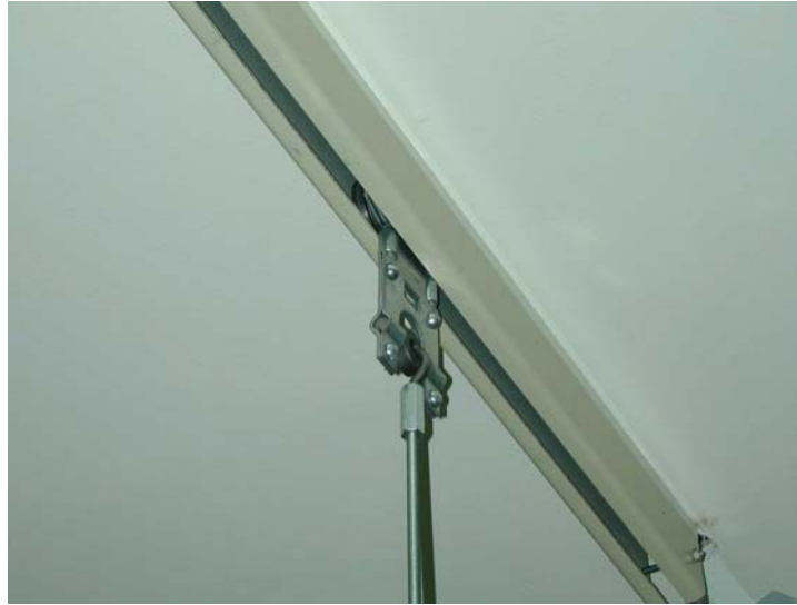
Figure 3.1 – Rail Track in Ceiling
