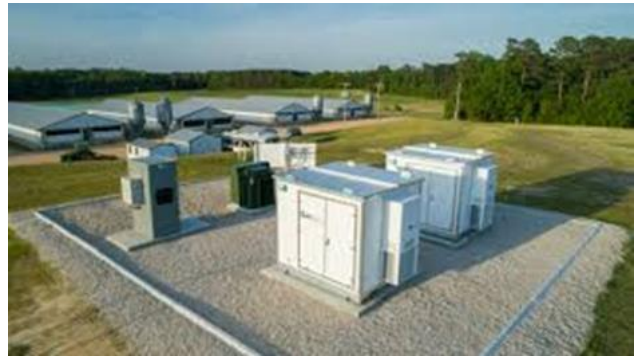
Butler Farm Microgrid – White Oak, NC (Appendix 3: Butler Farm Microgrid)
