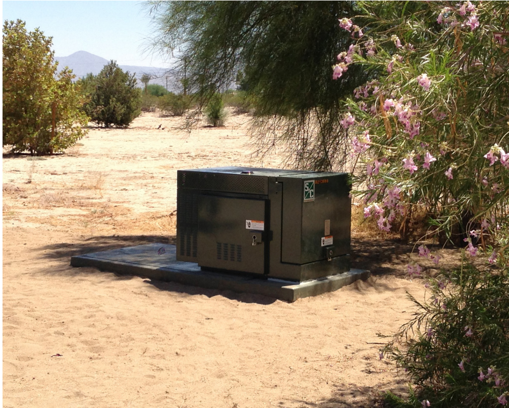
Photo Courtesy S&C Electric
