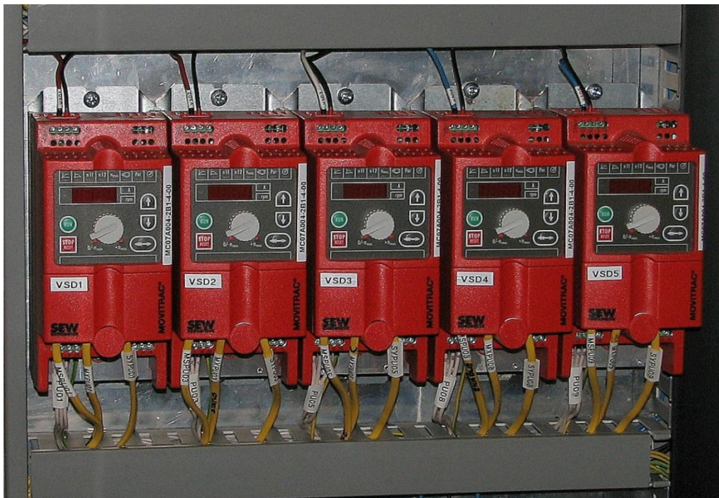
Figure 30 UWS SEW Variable Speed Drives
