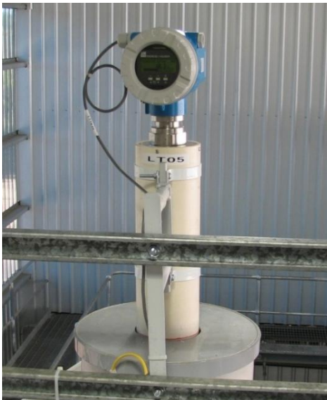
Figure 21 Tank 05 Micropilot M Radar Level Transmitter
