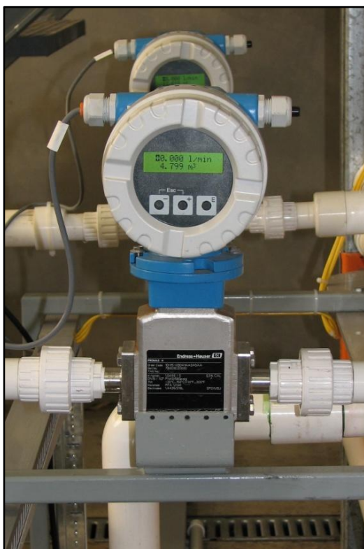
Figure 24 Promag M Magnetic Flow Meter FIT02
