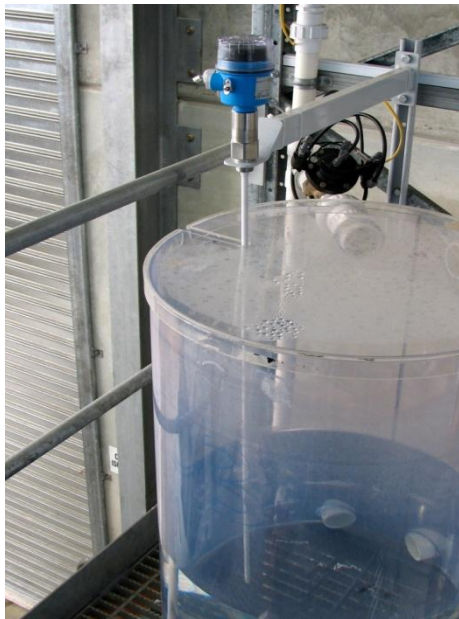
Figure 19 Tank 03 Liquicap M Capacitance Level Transmitter
