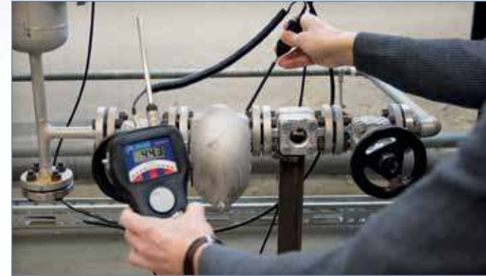
Steam trap testing and energy audits
