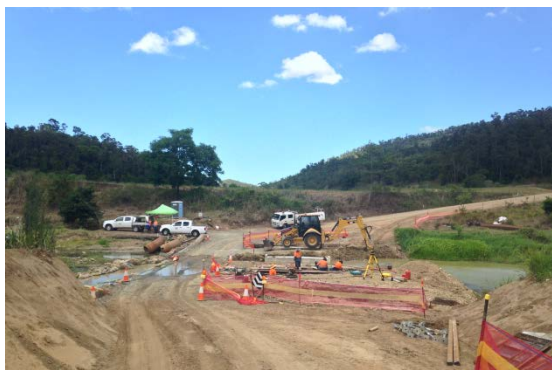
Murray Creek – Existing causeway on the left, new bridge construction on the right
