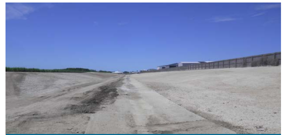
Monash Way – Completed drain with concrete invert. Note that the sides of the drains are hydro mulched to promote vegetation growth giving the white appearance.
