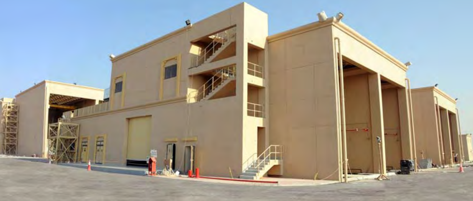
Civil & Building Works - Control and SCADA Building of Dubai Land II- 400/132 kV Substation
