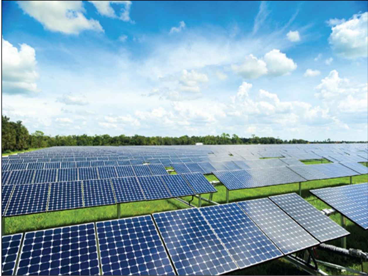
Photo 3.8-2. Single-axis, tracking photovoltaic system with panels close to maximum tilt
