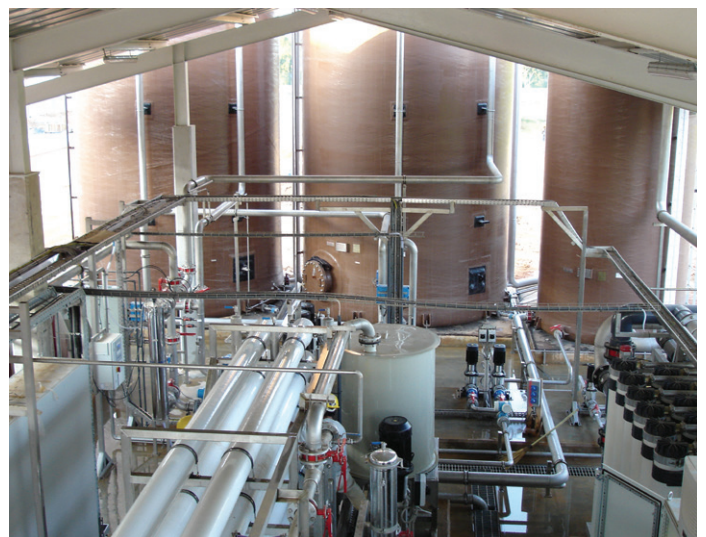
Heineken, Laos, water reuse AQUALITY® ultrafiltration - EXSEL® reverse osmosis Water reuse: 317,000 ft 3 /d
