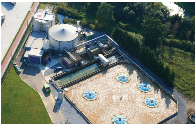
Danone, Belgium - BIOTIM® UASB Capacity: 15,070 lbs COD/d - biogas: 71.960 ft³/d
