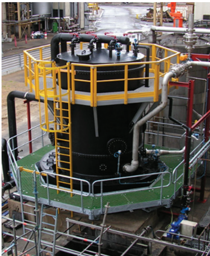
Cargill, Belgium, sulphur removal from extraction gas 4 -stage BELGAS® scrubber Flue gas flow: 7,000 ft 3 /h
