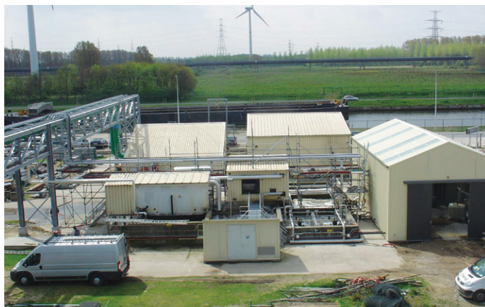
Cargill, Belgium ATLANTIS® submerged MBR - 4,400 lbs COD/d
