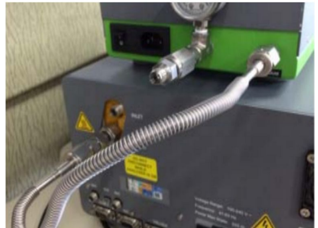
Figure 4 External recirculating pump with CVR coupling and Swagelok fitting attached.
