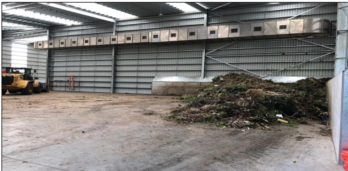
Figure 13 - Inside Receiving Building with Air handling Ducts- Shell Harbour NSW Invessel Compost Facility
