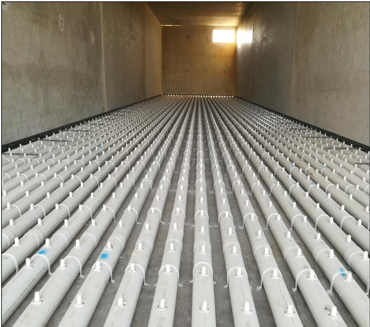
Figure 16 - Aeration Tunnel Floor Air Pattern Design - Yatala QLD. Invessel Compost Facility
