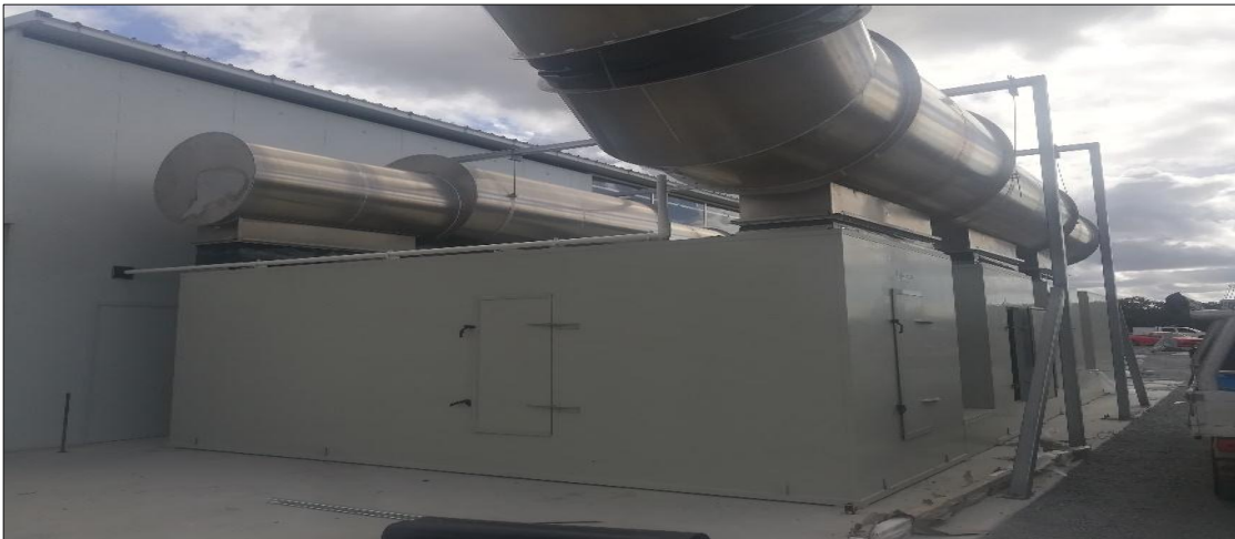
Figure 25 - Chemical Scrubber - Yatala QLD. Invessel Compost Facility
