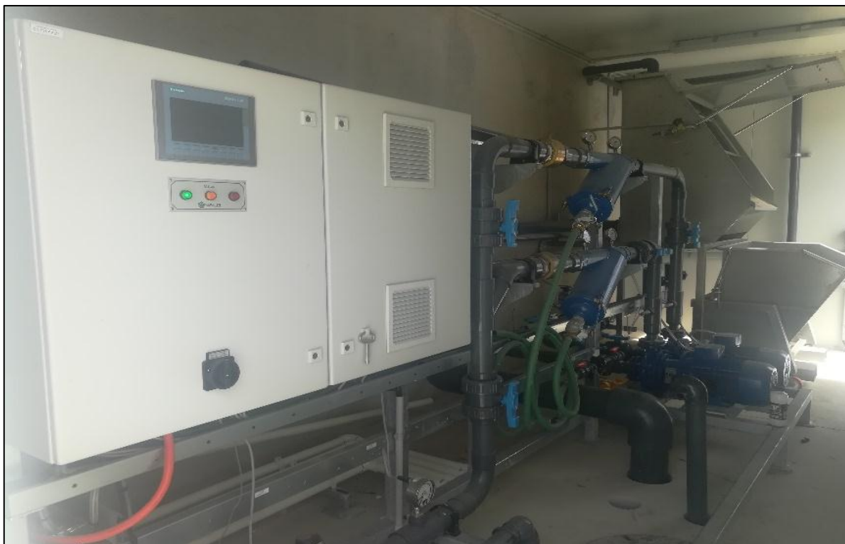
Figure 40 - Leachate Re-Use Pump Room – Shell Harbour, NSW
