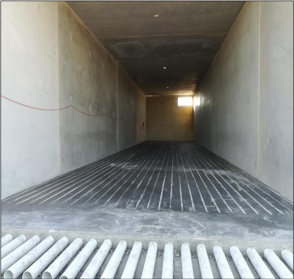
Figure 17 – Finished Aeration Tunnel Floor with Leachate Collection Pipes- Yatala QLD. Invessel Compost Facility
