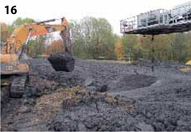
The clayshale rock was transformed into a mud by large quantities of water added to the cutterhead
