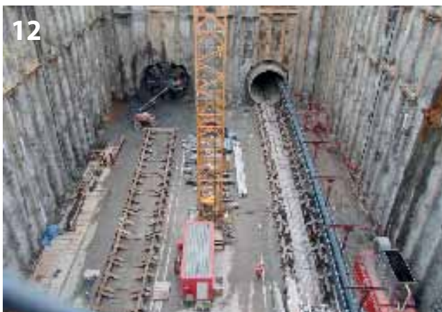
a) Steel cradle in a curve prepared for the shield in the intermediate shaft
