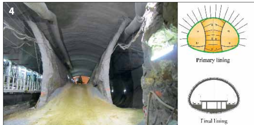
Station excavation implemented the twin side-wall drift method, which first built the side drifts to support the station arch. The left side drift shows the EPBM gantry
