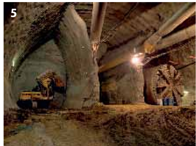
The side-drifts of Petrín Station were filled with light concrete to form a vertical wall for the EPBM breakthrough
