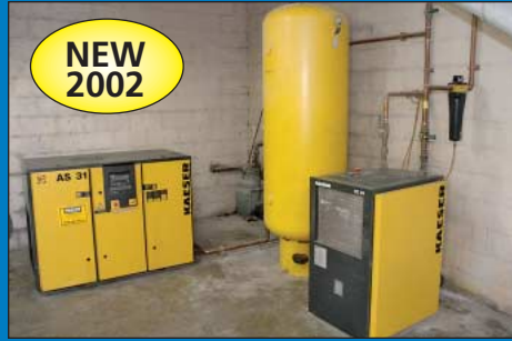
Overall View Air Compressor System Including 25 HP Kaeser Model AS31 Compressor, Dryer and Tank
