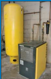
Close Up View Dryer and Tank
