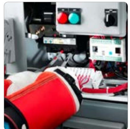
...for example circuit-breaker testing
