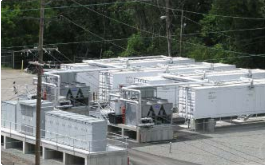
IEC TC 120: Electrical energy storage systems, aims to help make energy supply more efficient through standardization for EES (Photo: AES Energy Storage)
