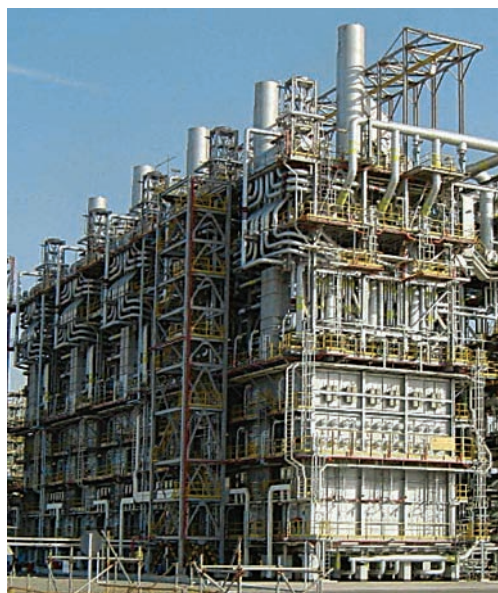
Figure 5. Furnace section of a modern ethylene plant
