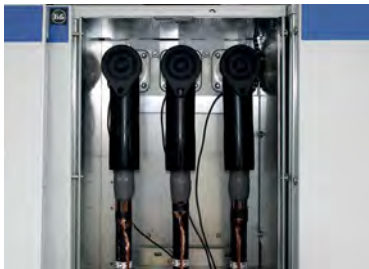
SF-6 system connection with 480TB
