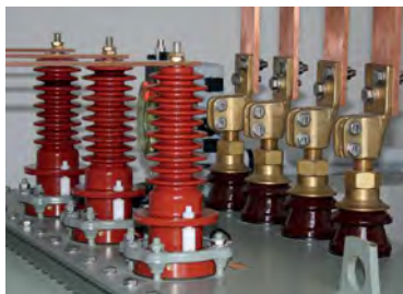
PITO-E on transformer with bushings
