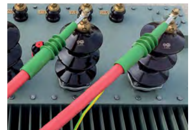
AIP20 as a transformer connection
