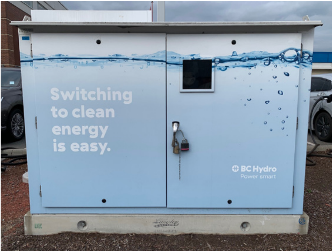
Figure 1: BC Hydro kiosk for EV charging station
