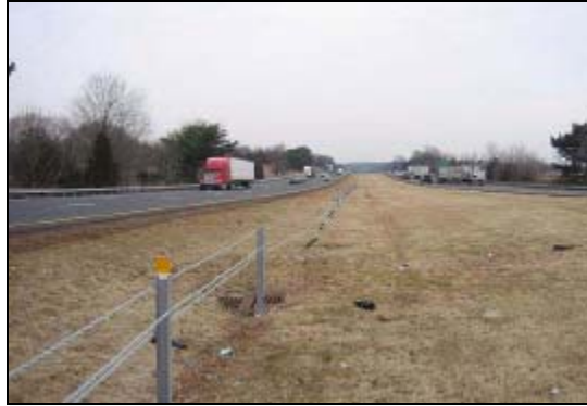
Figure 35. Impact 2: Barrier Damage
