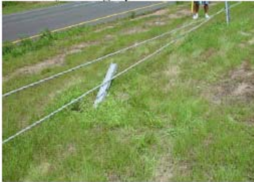
Post 3 bent, tire tracks visible
