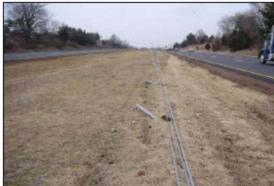
Figure 34. Impact 1: Barrier Damage
