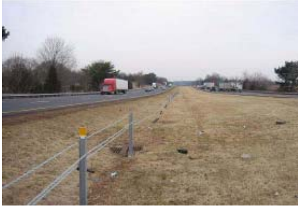
TOPLEFT: Front view of the damaged section of barrier, facing East.
