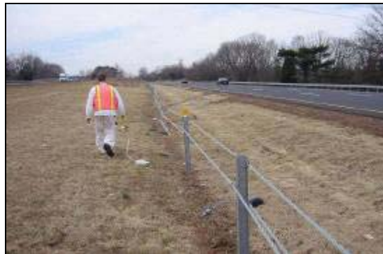
Figure 36. Impact 3: Barrier Damage
