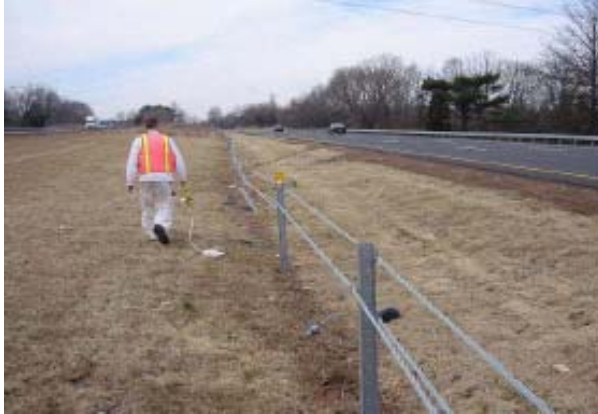
TOPLEFT: Front view of the damaged section of barrier, facing West.
