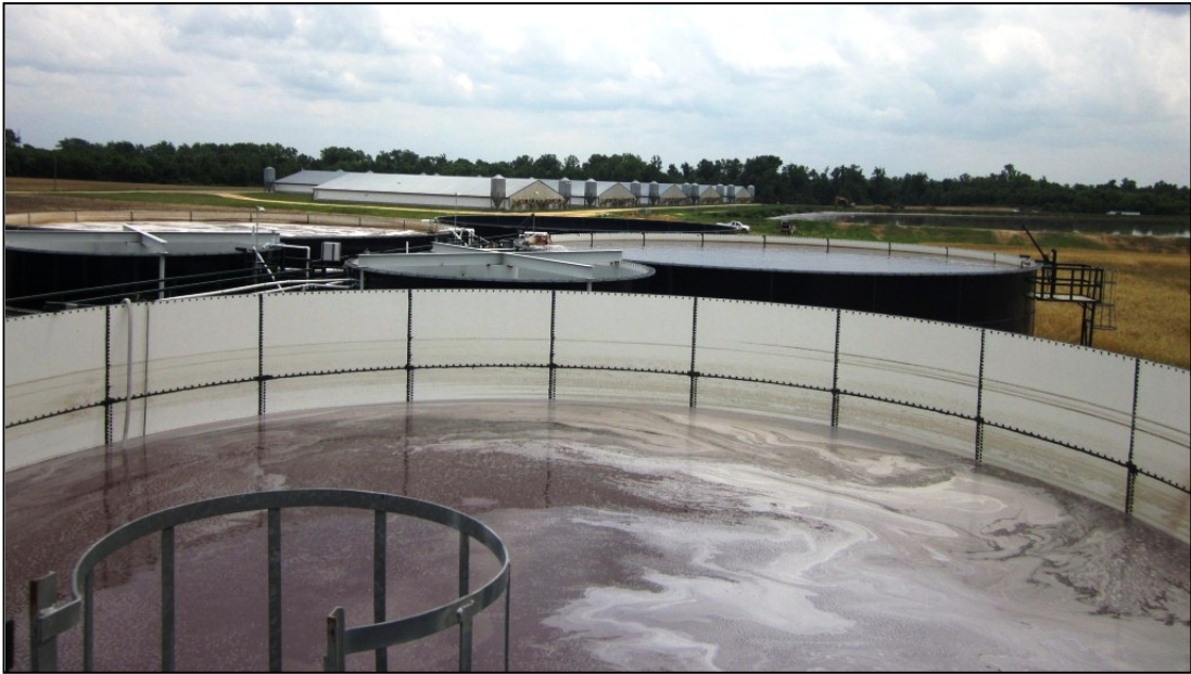
Separated water tank; it is placed after solids separation and before N module.
