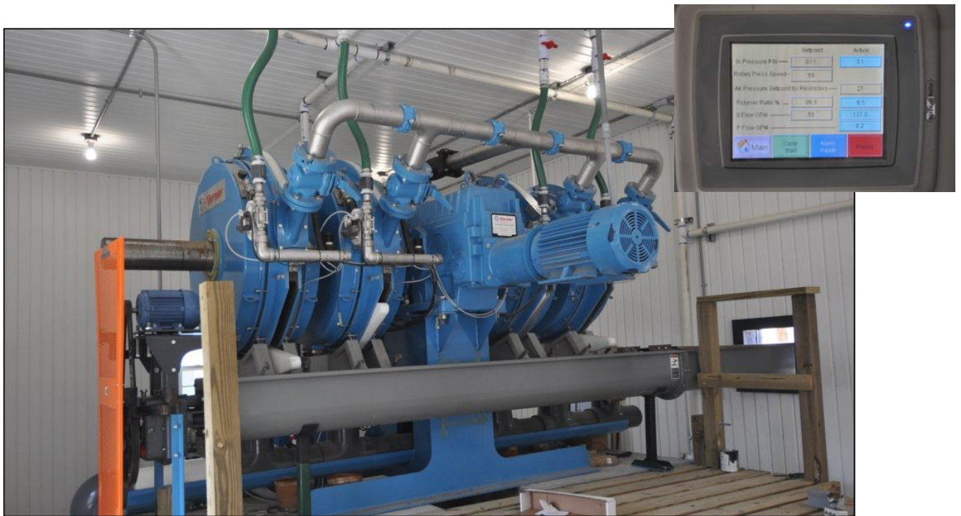
Rotary press used for solid-liquid separation. Touch-screen process control is shown in upper right photo.
