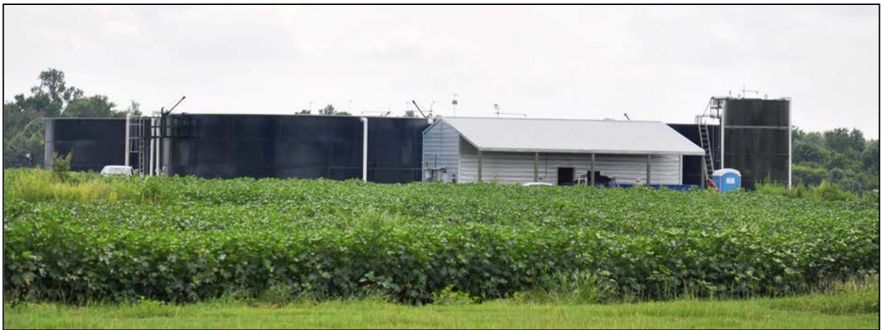
View of manure treatment system at Jernigan farm. Building contains the solid-liquid separator. Tanks at left are homogenization tank (front) and nitrification tank (back); tall tank at right is decanting tank.
