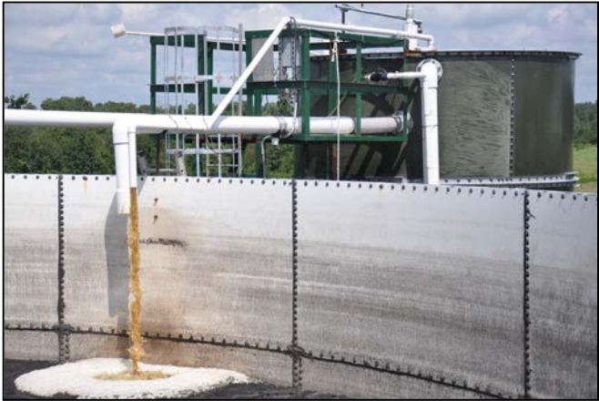
Decanting tank, clarified effluent, and sludge sampling
