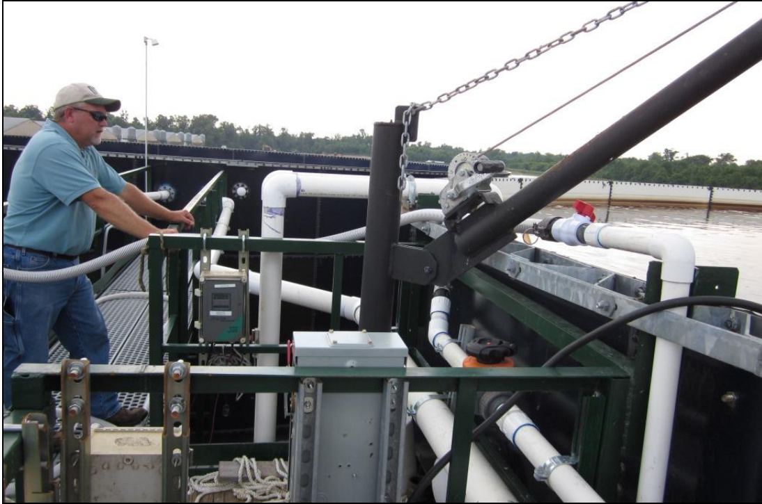
Denitrification tank hoist that supports submersible mixer.
