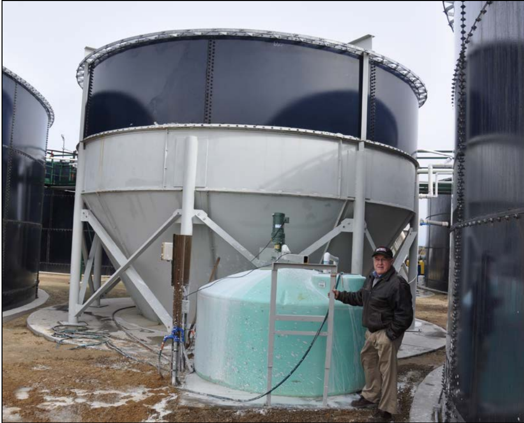
Lime preparation tank (green) and settling tank used in the phosphorus removal module.
