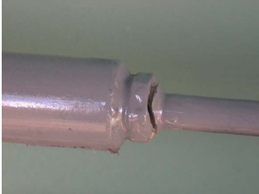
Figure 12. Slip between the CFRP bar and the steel tube anchor interface.
